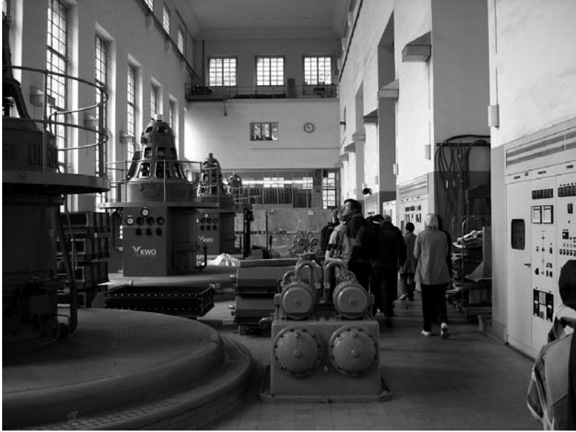
Fig. 6: Visitors at Powerstation Handeck 1: hall with turbines and generators (Photo Bernhard Gunzenhauser).
